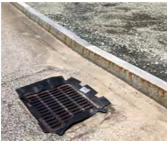
Protect storm drain inlets
