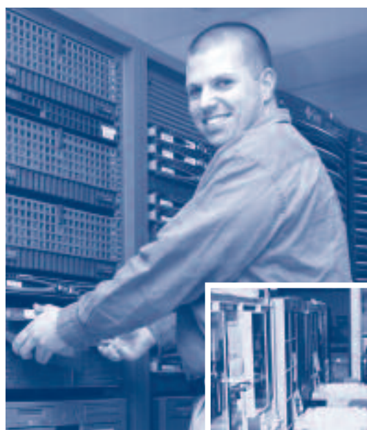
Systems Administration Engineer Sean Frenette installing a server in the Data Center.
