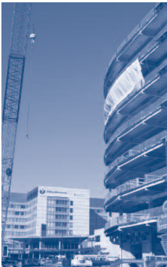
Design of the Advanced Center for Clinical Education and Science incorporates enhanced energy performance, sustainable site design, recyclables collection and storage, and low-emitting paint and carpets.
