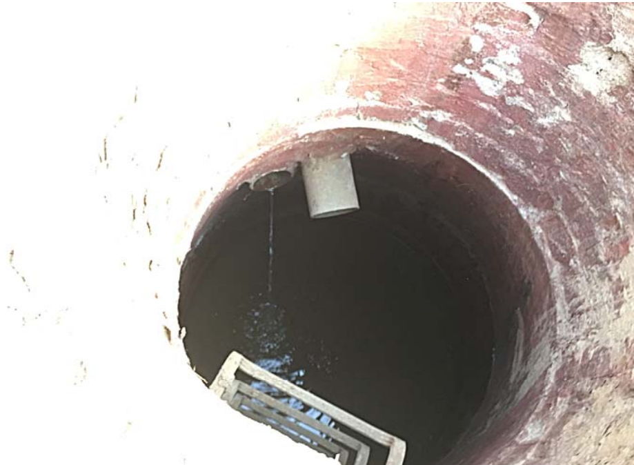
Flow Observed From Drain to Tank
