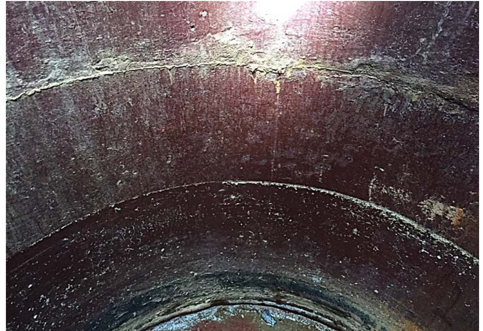
West Tank Side Wall. High Level Water Mark Near Tank Bottom
