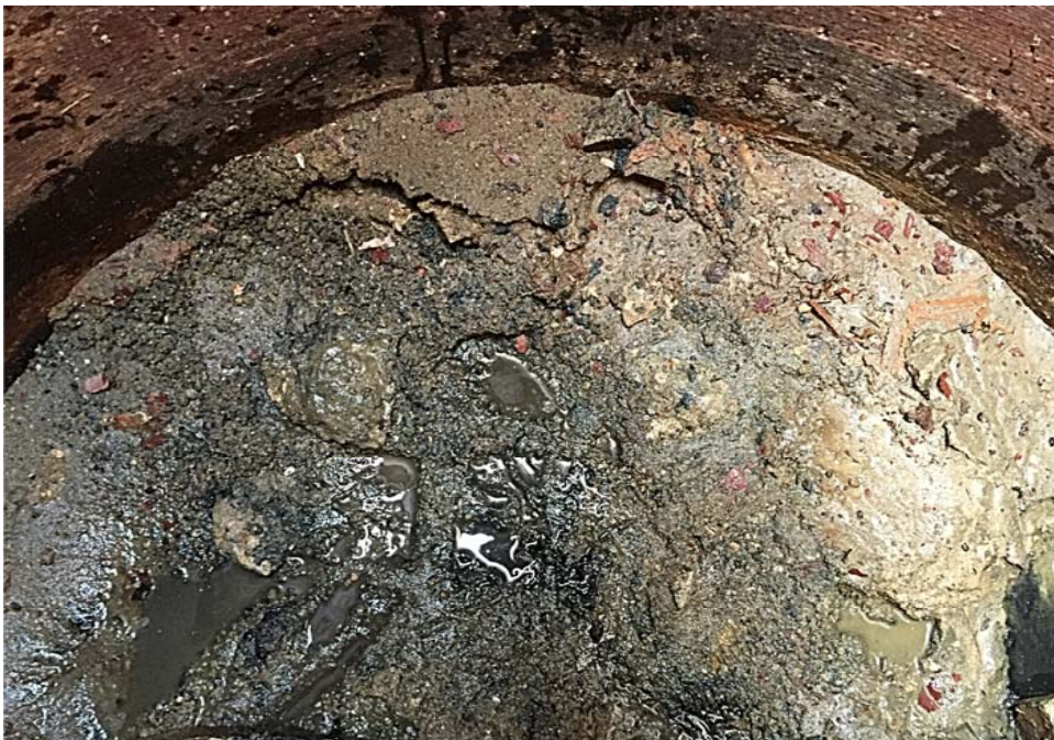
East Tank Bottom Following Liquid Removal. Sediment Remains
