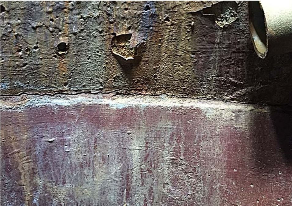
West Tank Sidewall. Crack Observed at Seam
