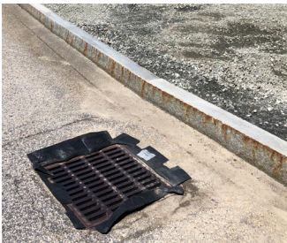
Protect storm drain inlets
